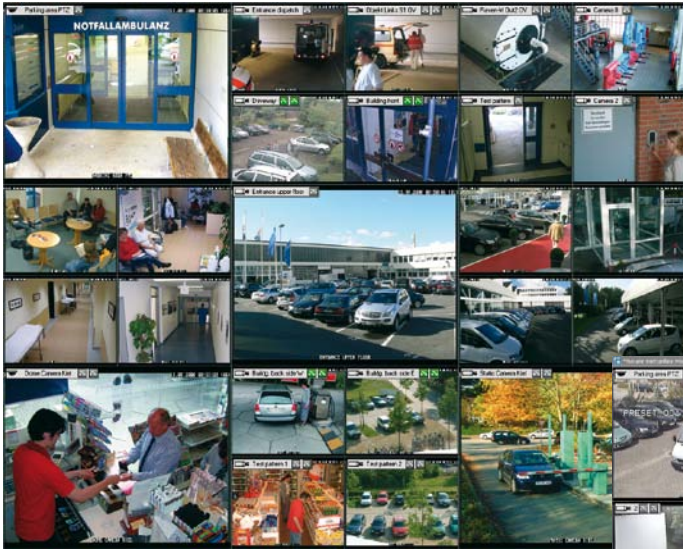
CamControl MV monitor with display of 24 cameras and freely definable layout on up to 4 monitors.
